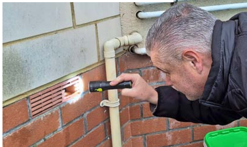
> Checking for rats through a hole in an outside vent
